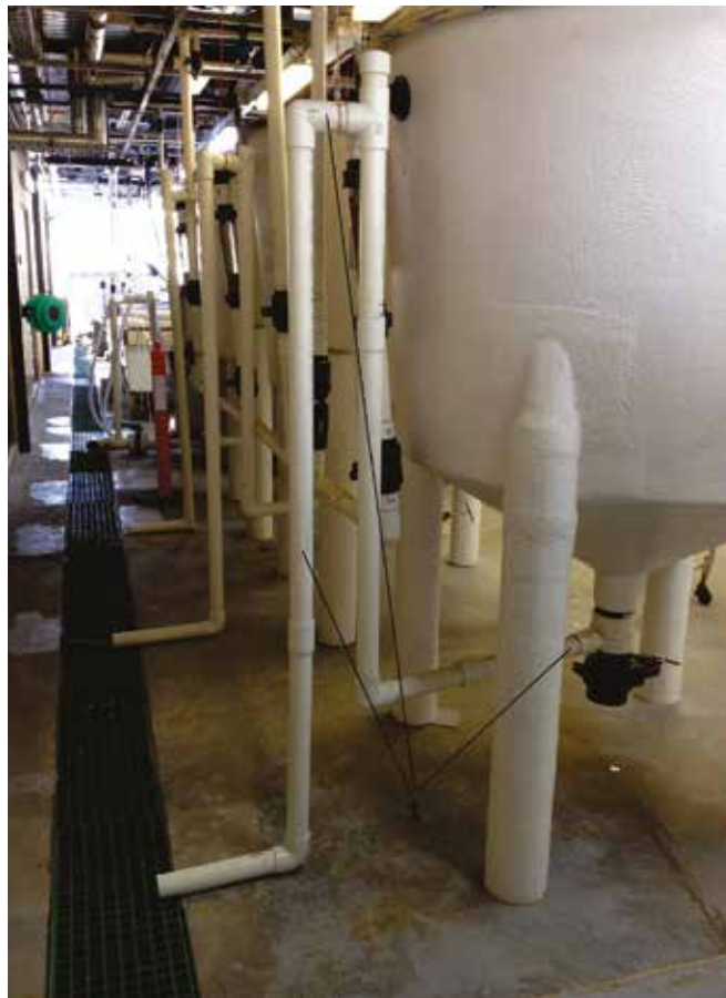
Figure 18. External Standpipe (1) attached to the base of the tank.
