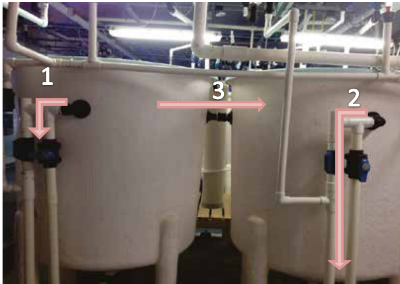
Figure 59. External standpipe with valve closed in existing tank during transfer (1), preventing water from overflowing and directing it to the tank connection (3), external standpipe with valve open, allowing normal overflow in new tank (2).
