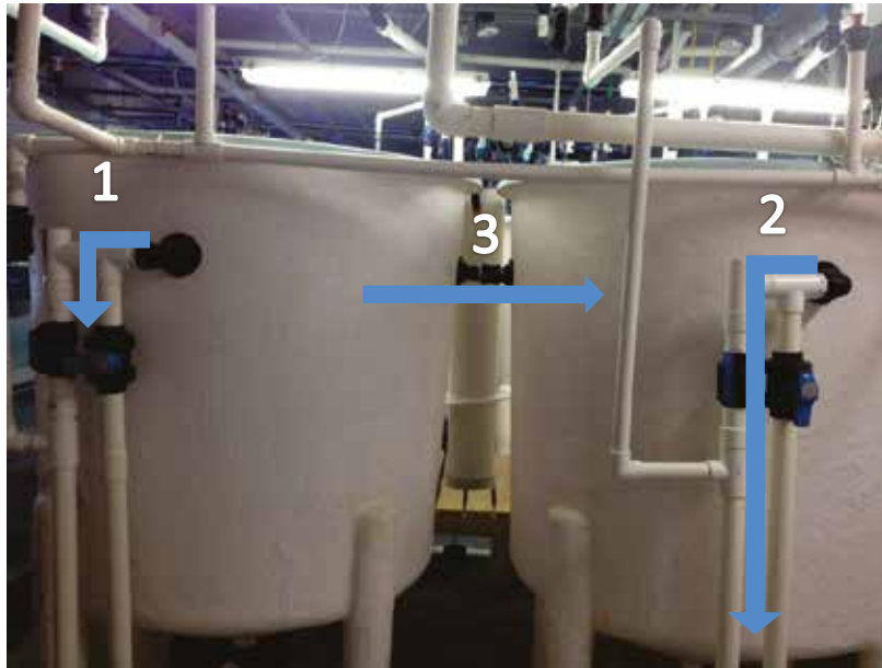
Figure 43. External standpipe with valve closed in existing tank during transfer (1) preventing water from overflowing and directing it to the tank connection (3) external standpipe with valve open, allowing normal overflow in new tank (2)
