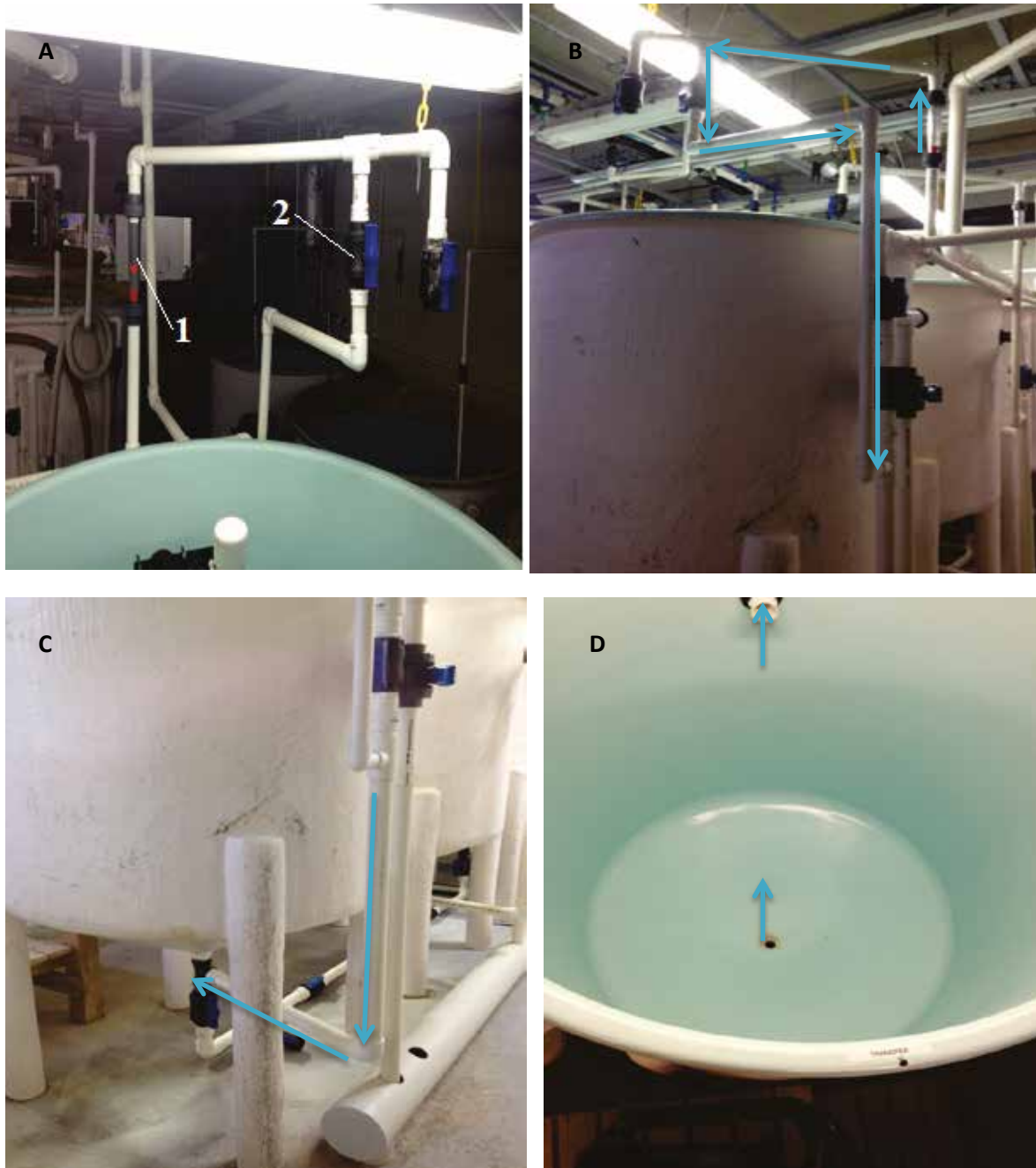
Figure 32. A. rotameter (1), seawater inlet valve (2), B. water entering external standpipe, C. water entering at the tank bottom, D. water entering up through the base and exiting the top of the tank. Blue arrows represent water direction.
